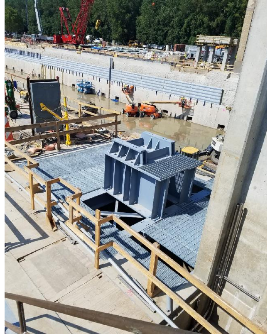
New gate machinery base
